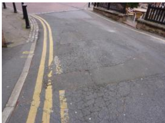
Photograph 44: Poor quality Tarmac on Denmark Street
